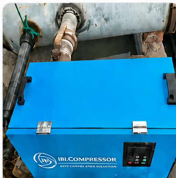
A After Retrofit: IBI High-Speed Centrifugal Blower On Site
