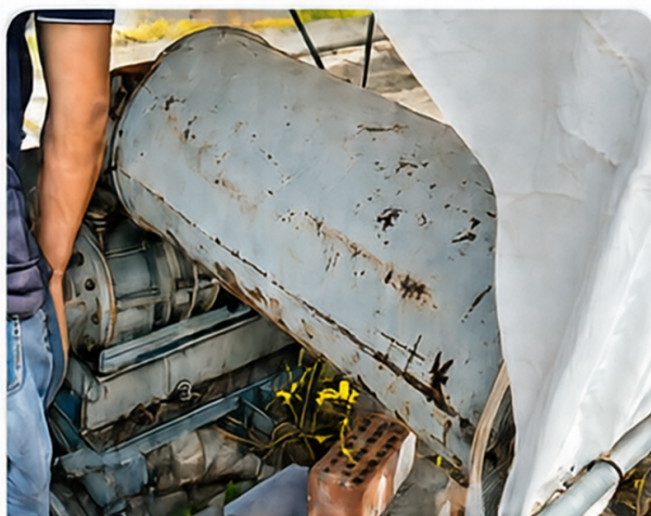
B Before Retrofit: Original Roots Blower On Site
